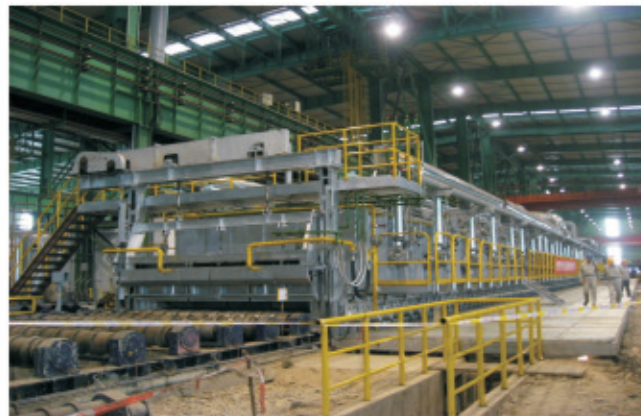
Heat Treatment Line for Medium Plate Mill of Xinjiang Bayi Steel, Baosteel (EPC)
