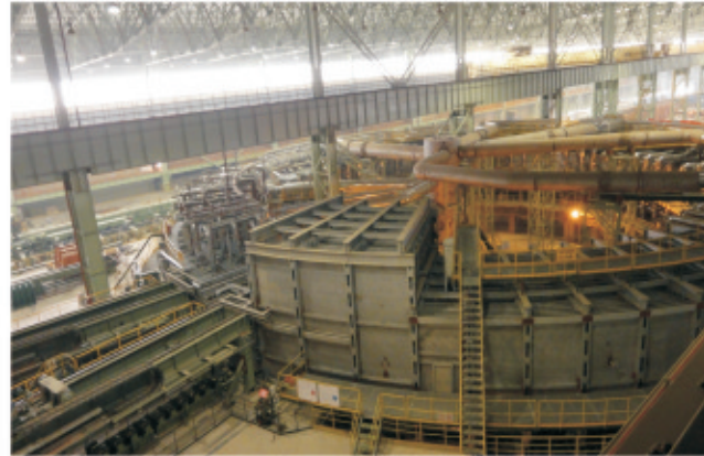
Φ 50m Rotary RHF for Continuous Tube Mill of Lubao Steel Pipe (EP) —China's Largest Rotary RHF so far
