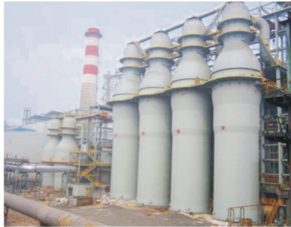
Top-combustion Hot Stoves
