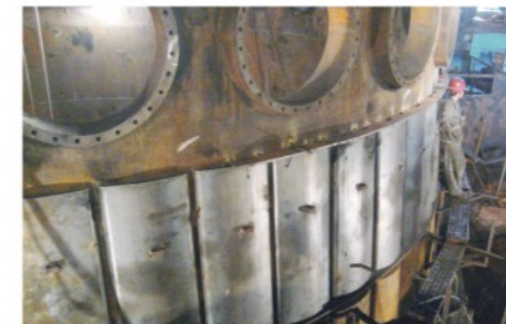
Trough plate cooling equipment
