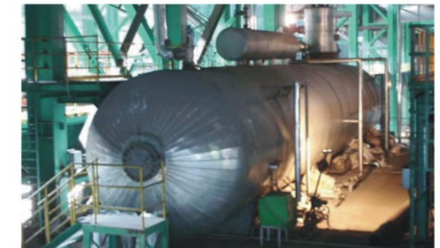
Micro-superheat Recuperator in Operation
