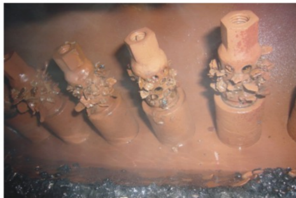
Boiler Failure due to Poor Circulating Water Quality
