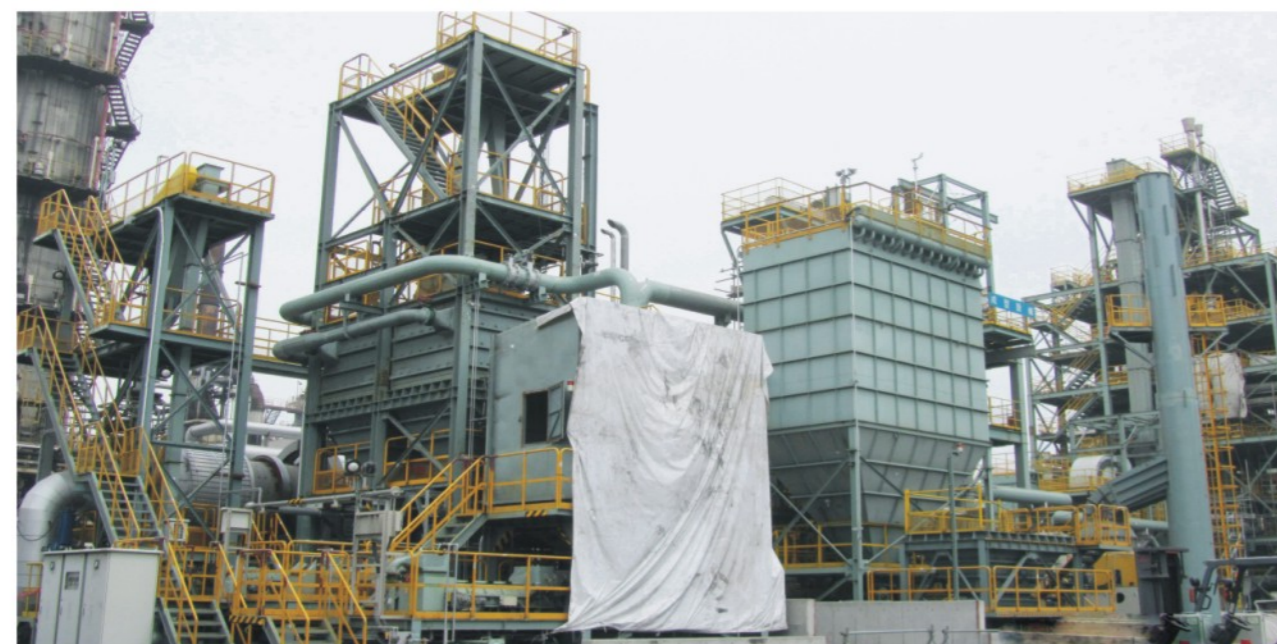
Ferrocoke Raw Material Handling & Storage Equipment
