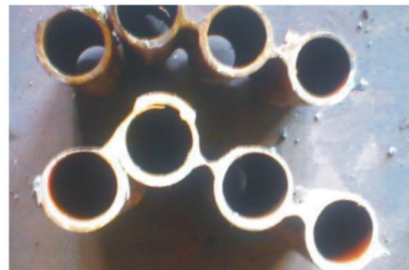
Boiler Failure due to Non-uniform Circulating Water Distribution
